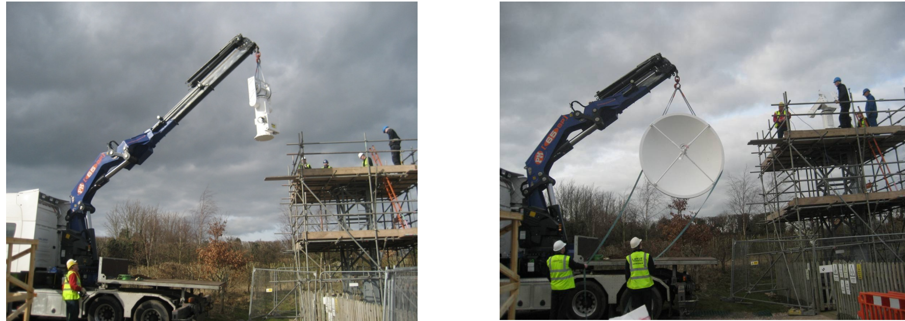
Figure 1. Upgrade of the Met Office direct broadcast reception facilities at Exeter HQ.
