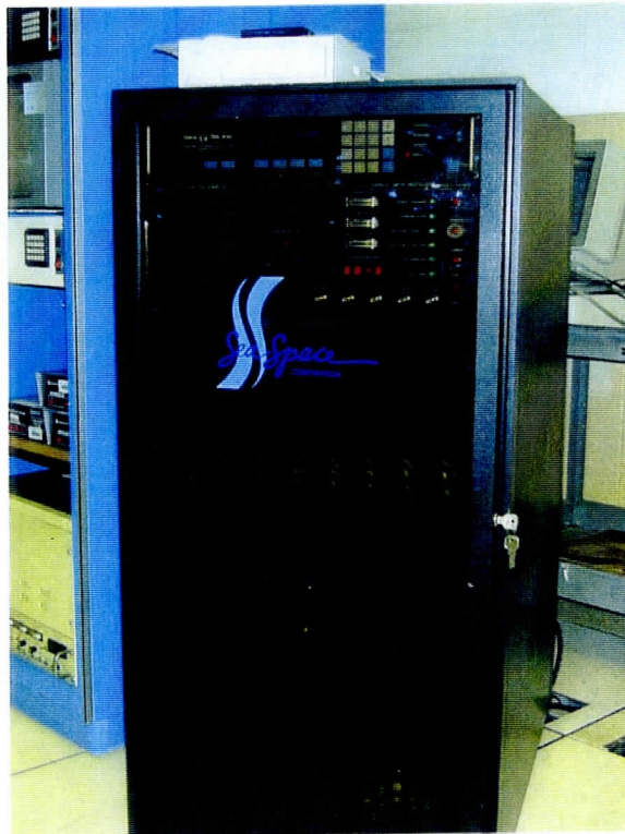
Figure 4: SeaSpace equipment rack (antenna controller, receiver, control computer, UPS)
