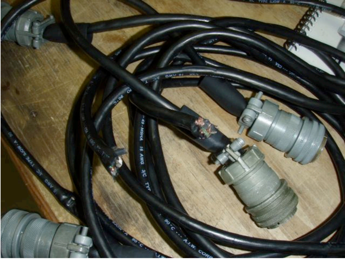
Image A2: Damaged battery cables from Minna Bluff AWS
