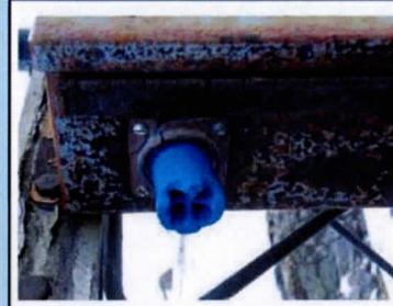
Junction box (Bad condition)
