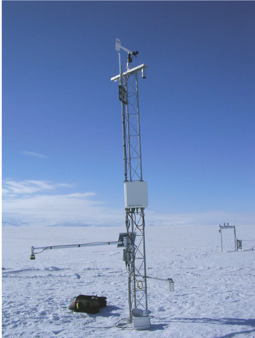
Image A31: New AWS 30477 after installation at Williams Field site in February 2009
