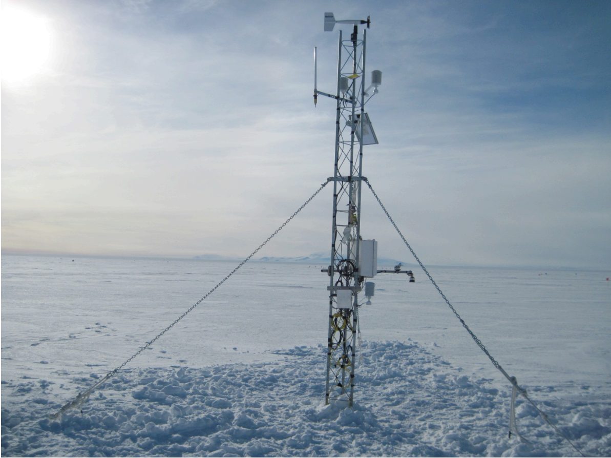
Janet AWS after installation on January 17 th , 2011
