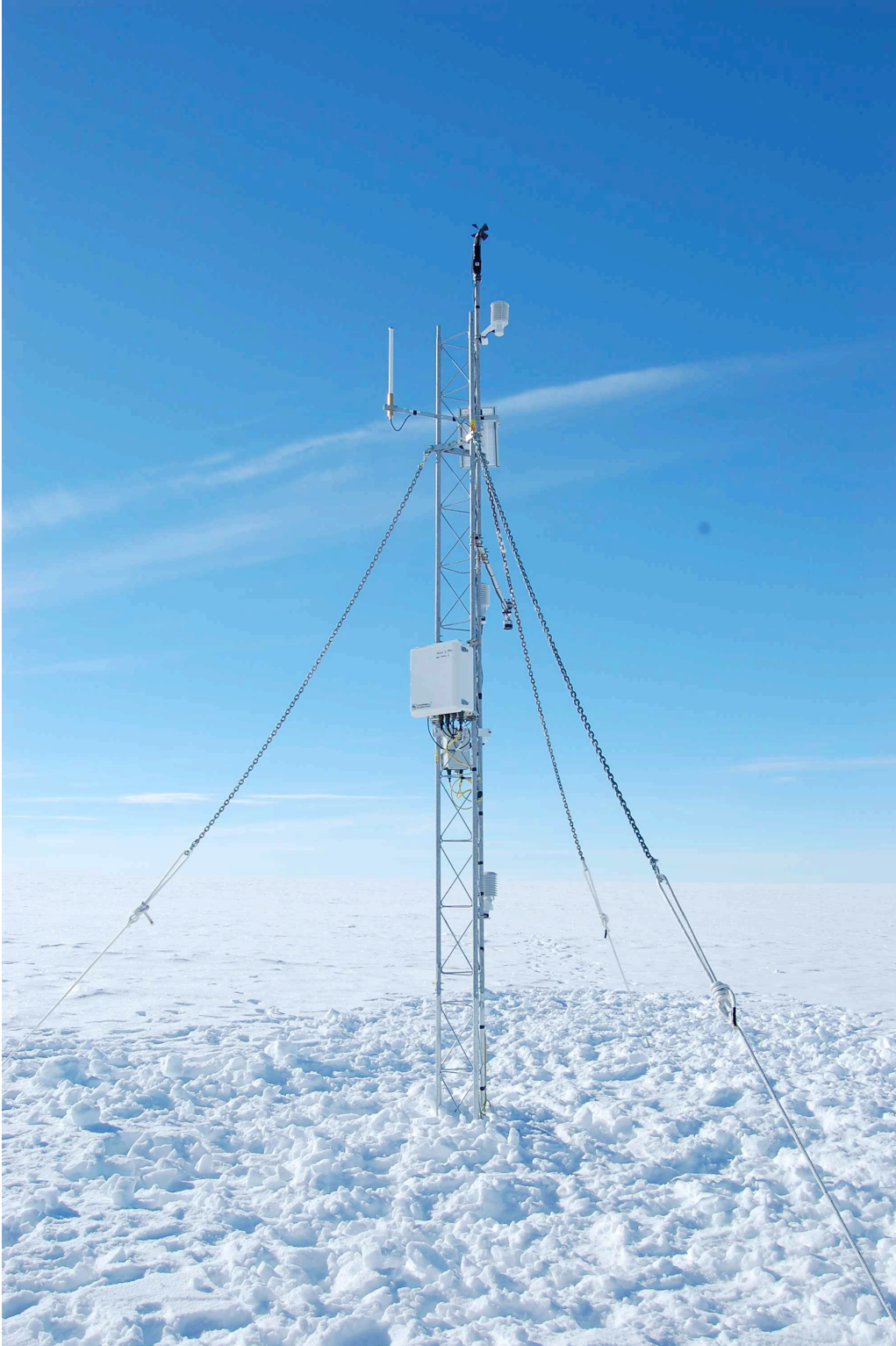
Marlene AWS site after installation on January 13 th , 2011
