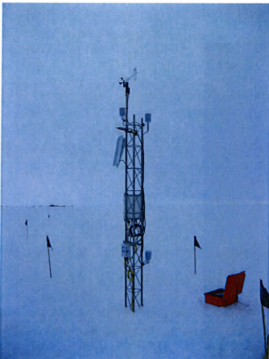
Willie Field after Freewave conversion
