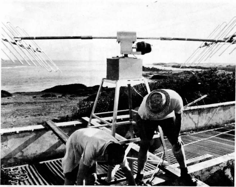
Figure 10. The APT (satellite receiving) antenna being installed on the BOMEX Operations Building on Barbados during May, 1969. This antenna is remotely controlled by operators within the building using computer computations of the orbital position of the satellites. The ESSA satellites in 0900 and 1500 local time orbits were read-out daily, as well as the NIMBUS III satellite at noon and midnight local time. Pictures were also received from the ATS-III satellite which was nearly stationary over Barbados but drifting slowly eastward during the BOMEX observation period.
